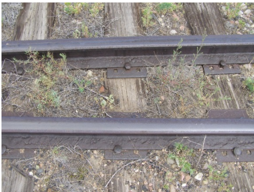
Spalling of Rail Flange
