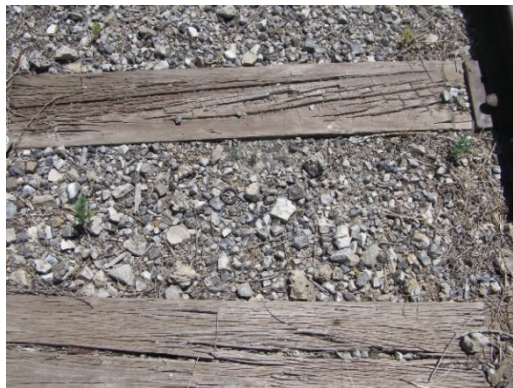
Deteriorated, small, well graded ballast
