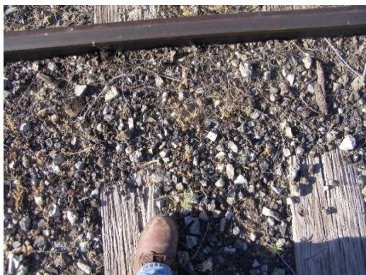
Typical Fouled Ballast in Classification Yard
