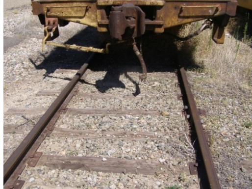
Warehouse Area Lowered Track, No Drainage
