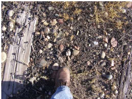
Typical Fouled Ballast in Classification Yard
