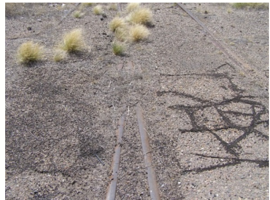
Warehouse Area Paved Track Deterioration
