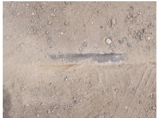
4 th Avenue Track Earthen Crossing Rail Corrosion
